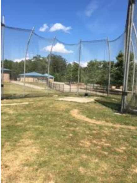
hammer cage with the non-functioning doors
